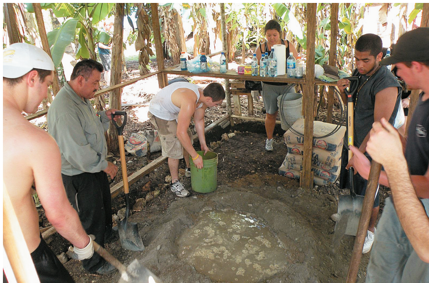
Northeastern University students help build a restaurant for Marina, a South African entrepreneur, as part of the Field Study Program.
